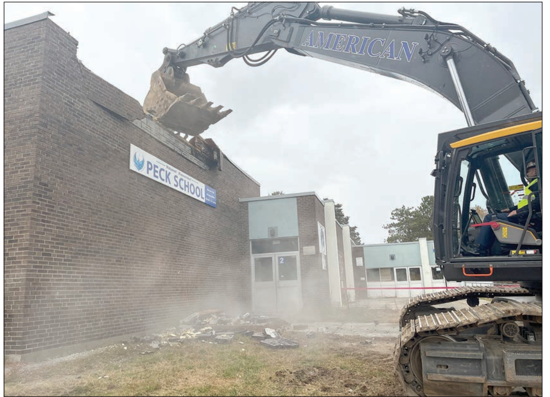
Funds were approved for multiple door and window replacements at city elementary schools. Work is also underway for the Peck Middle School project. Submitted photos
