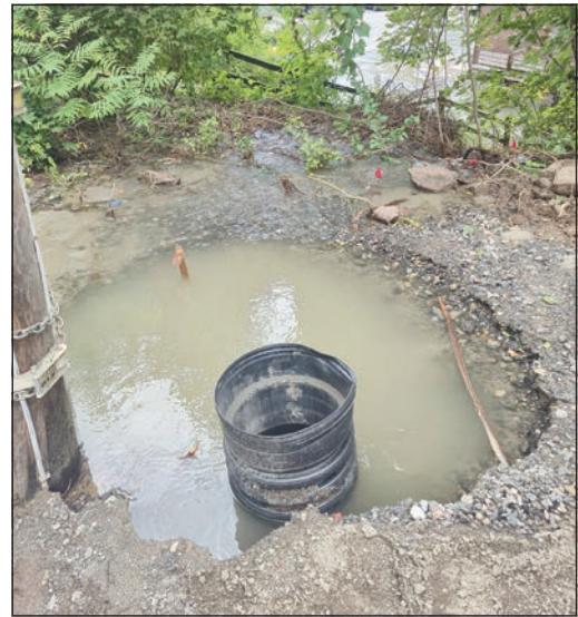
A pool of water formed after the leak.
