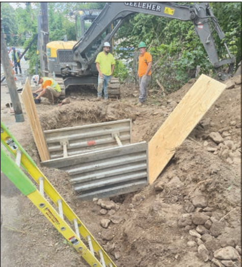
The broken water main is worked on Monday morning.
